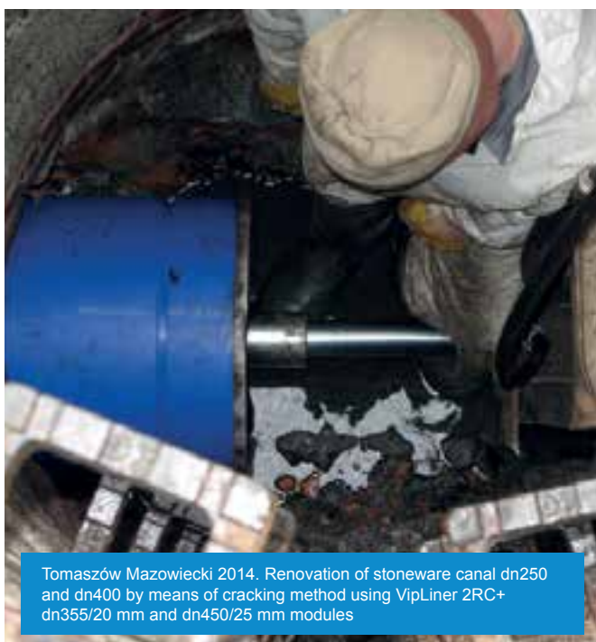
Ruda Śląska 2012. Renovation of storm water system with VipLiner dn200+630 mm modules
